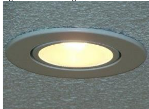
Gambar 10 Lampu Ruang Server
